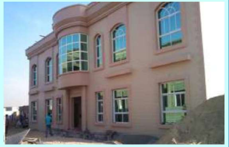
SECTOR : Z19, PLOT : 28 MBZ , CITY SCOPE : SUPPLY & INSTALLATION OF GLASS DOORS , WINDOWS & HAND RAILING
