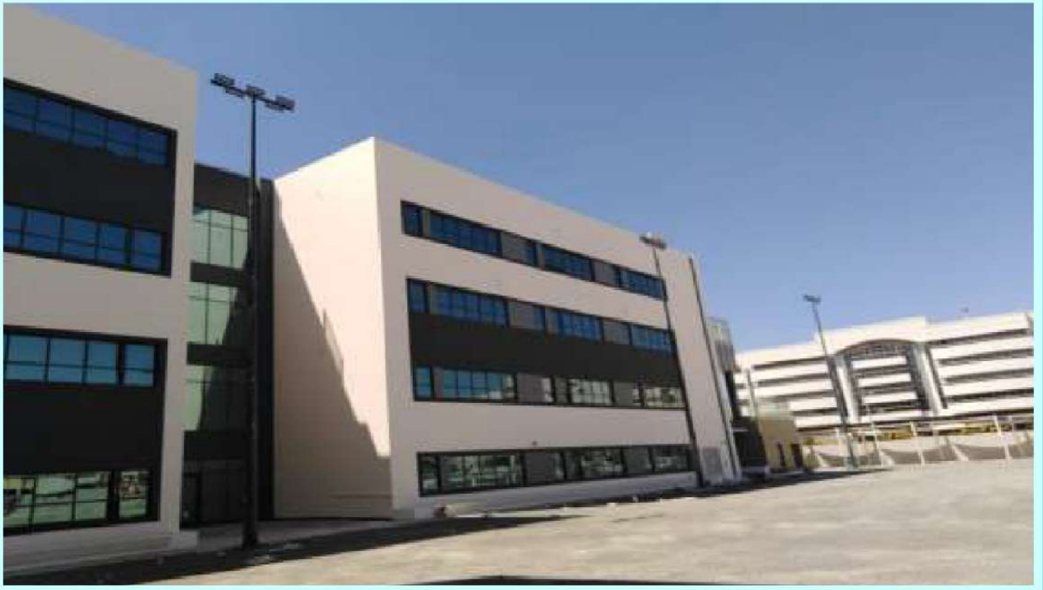
SECTOR : PEAR WISDOM SCHOOL, DUBAI SCOPE : SUPPLY & INSTALLATION OF GLASS CURTAIN WALL , DOORS ,WINDOWS, AND ALUMINIUM ACP CLADDING
