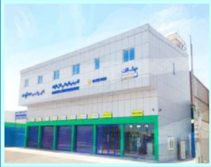
SECTOR : M7 MUSAFFAH COM BUILDING SCOPE : SUPPLY & INSTALLATION OF EXTERNAL ACP CLADING & WINDOWS
