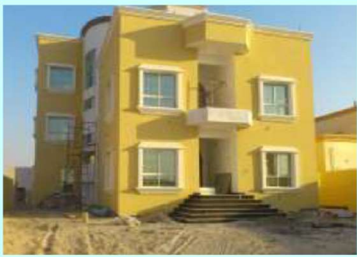
SECTOR : Z21, PLOT : 35 MBZ CITY SCOPE : SUPPLY & INSTALLATION OF GLASS DOORS , WINDOWS & HAND RAILING
