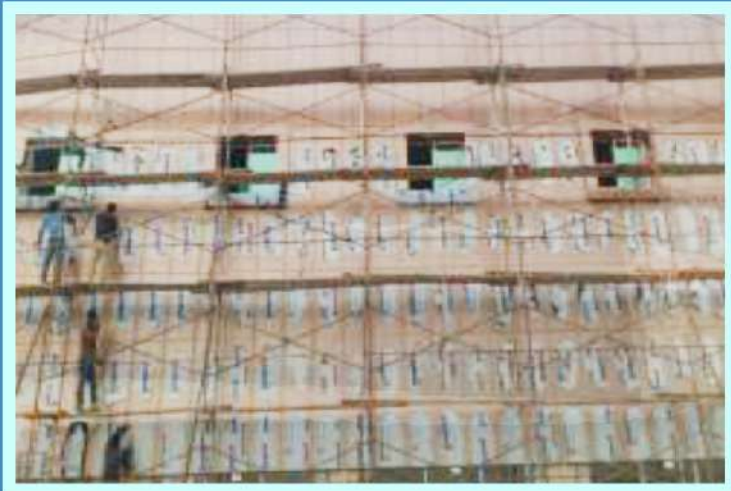
SECTOR : M37 MUSAFFAH COM BUILDING SCOPE : SUPPLY & INSTALLATION OF EXTERNAL ACP CLADING & WINDOWS
