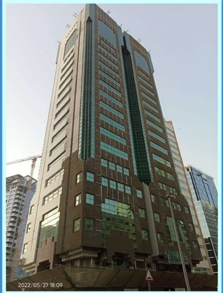
SECTOR : E13 , PLOT : C11, TCA SCOPE : REMOVAL EXISTING CERAMIC AND SUPPLY & INSTALLATION OF EXTRANAL ALUMINIUM ACP PANEL CLADDING
