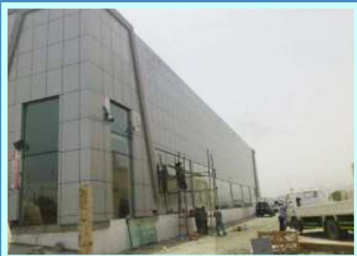
SECTOR : M10 MUSAFFAH COM BUILDING SCOPE : SUPPLY & INSTALLATION OF EXTERNAL ACP CLADING & WINDOWS
