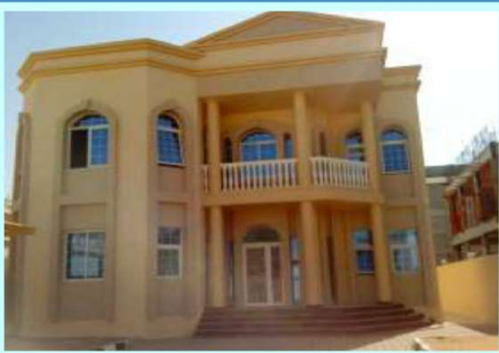
SECTOR : Z29, PLOT : 21 MBZ SCOPE : SUPPLY & INSTALLATION OF GLASS DOORS , WINDOWS & HAND RAILING
