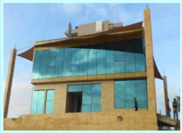
SECTOR : PRIVATE VILLA KCA SCOPE : SUPPLY & INSTALLATION OF GLASS CURTAIN WALL & WINDOWS
