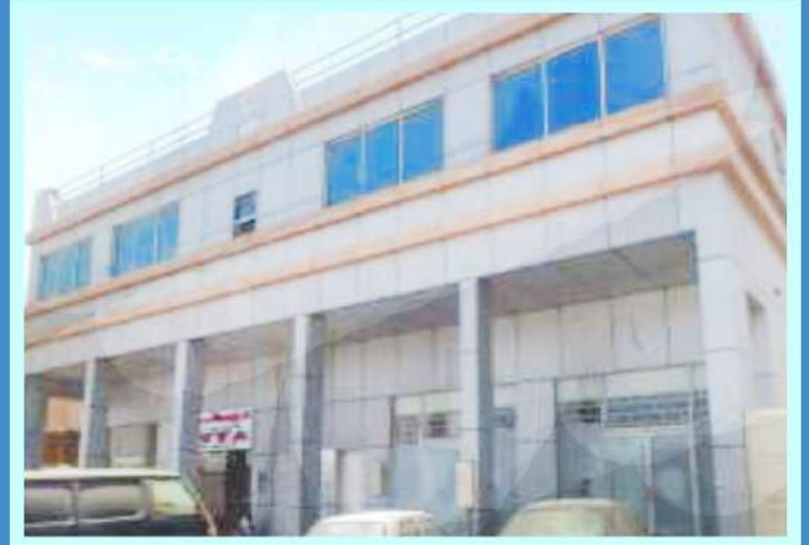
SECTOR : M13 MUSAFFAH COM BUILDING SCOPE : SUPPLY & INSTALLATION OF EXTERNAL ACP CLADING & WINDOWS
