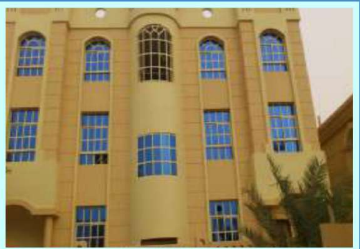
SECTOR : Z14, PLOT : 33 MBZ SCOPE : SUPPLY & INSTALLATION OF GLASS DOORS , WINDOWS & HAND RAILING
