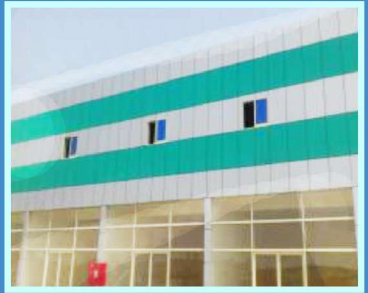
SECTOR : M36 MUSAFFAH COM BUILDING SCOPE : SUPPLY & INSTALLATION OF EXTERNAL ACP CLADING & WINDOWS
